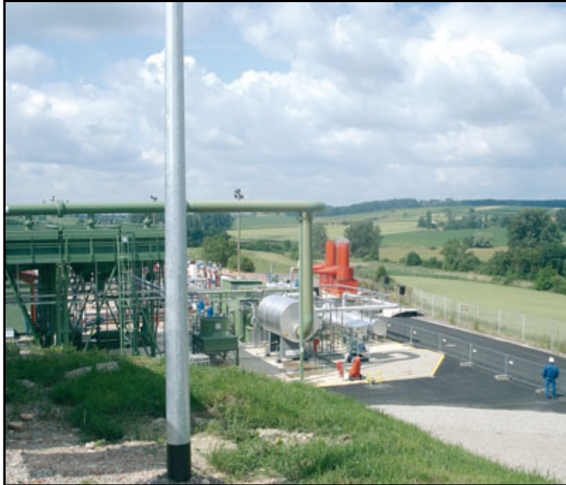
Figure 2: The Soultz geothermal power plant
